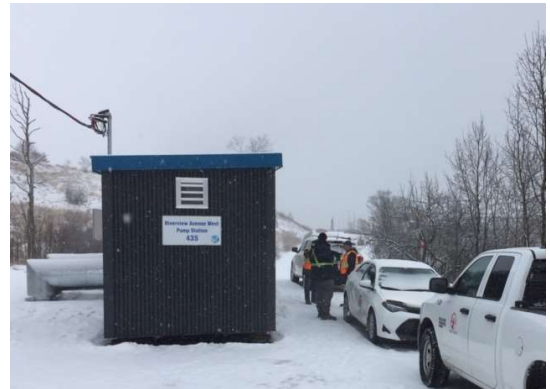
The new interim water pumping station supplying some west Saint John homes and businesses with water from the east side. (Photo: City of Saint John/Submitted)
