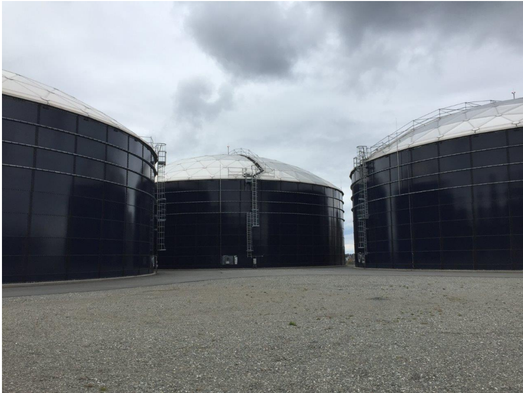
Three Water Storage Tanks (33ML Storage Capacity) At The Loch Lomond Drinking Water Treatment Facility
