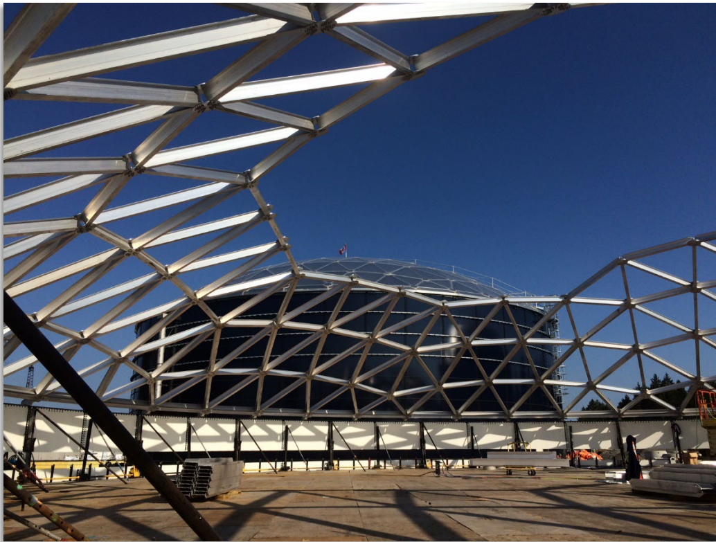
Water Tank Roof Construction At The Loch Lomond Drinking Water Treatment Facility
