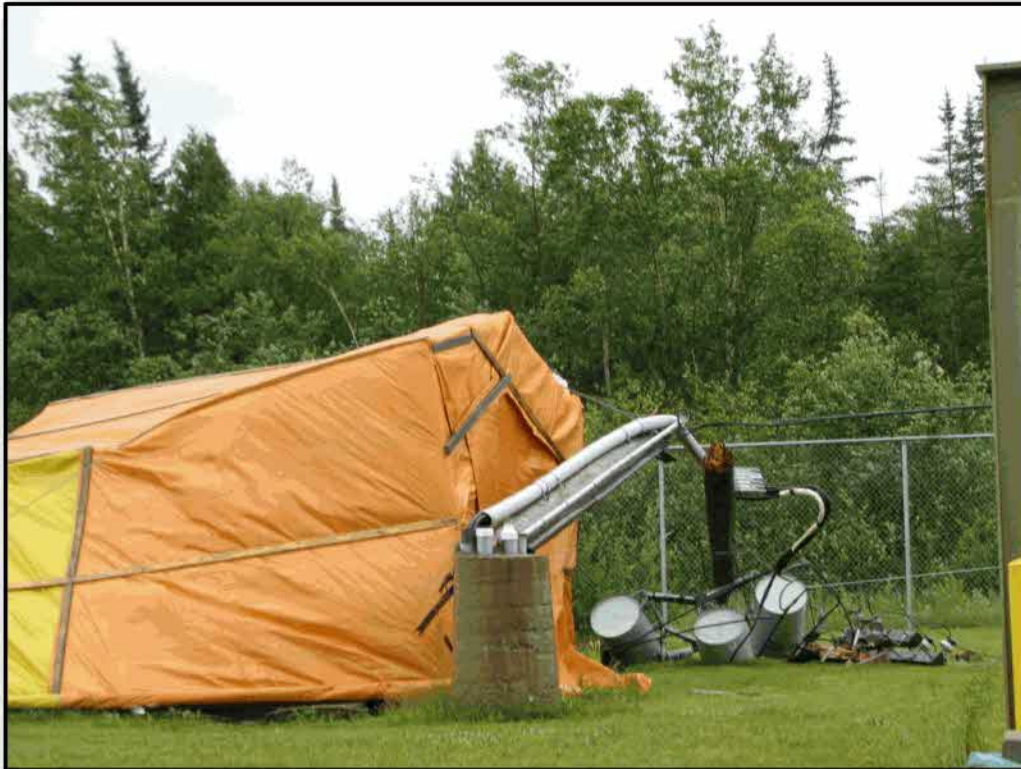
Latimer Lake Water Treatment Facility Electrical Pole Damage July 2014
